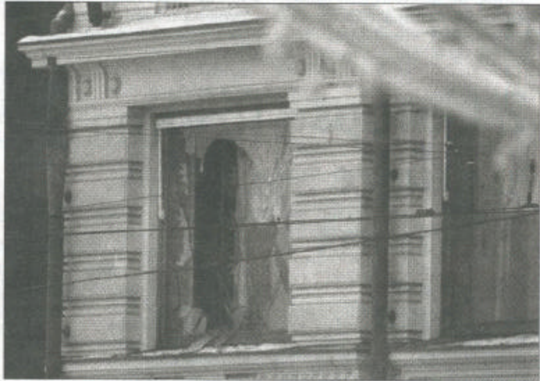
A second-floor window in the National Hotel that was broken by the force of the blast.
